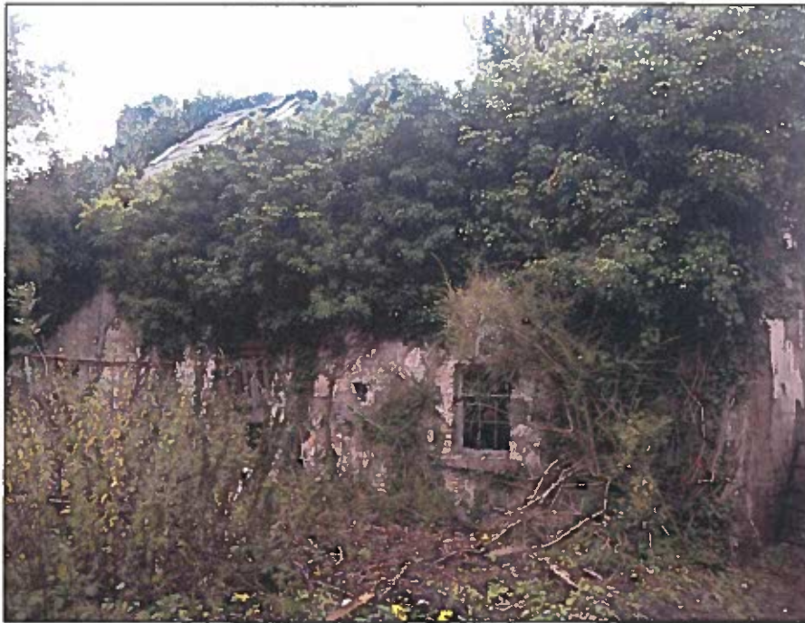
Figure 5: BL1 Stone Walls and Other Stonework - Old derelict building at 'The Hulk'.
